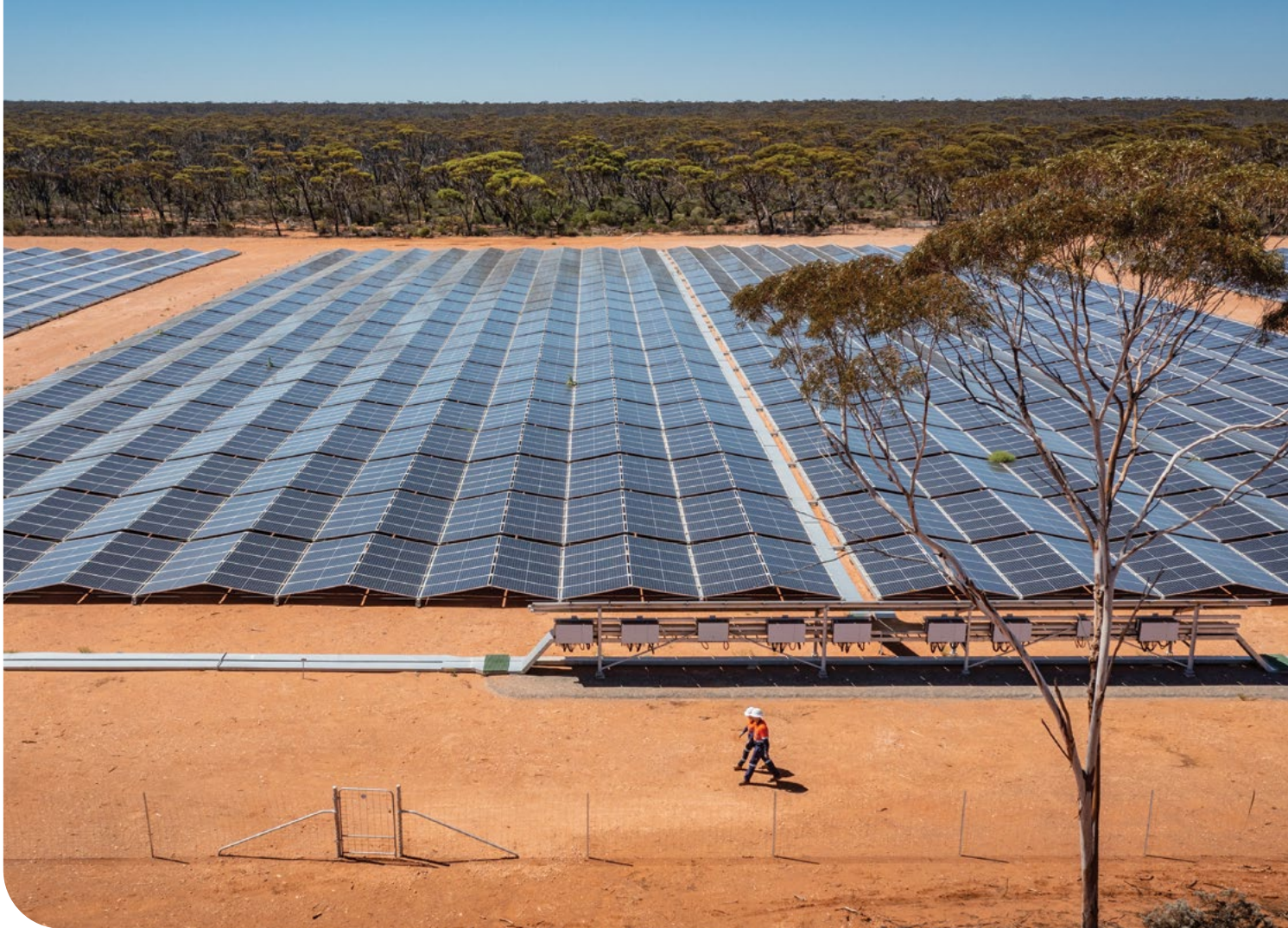
Image: Nova Operation solar farm
